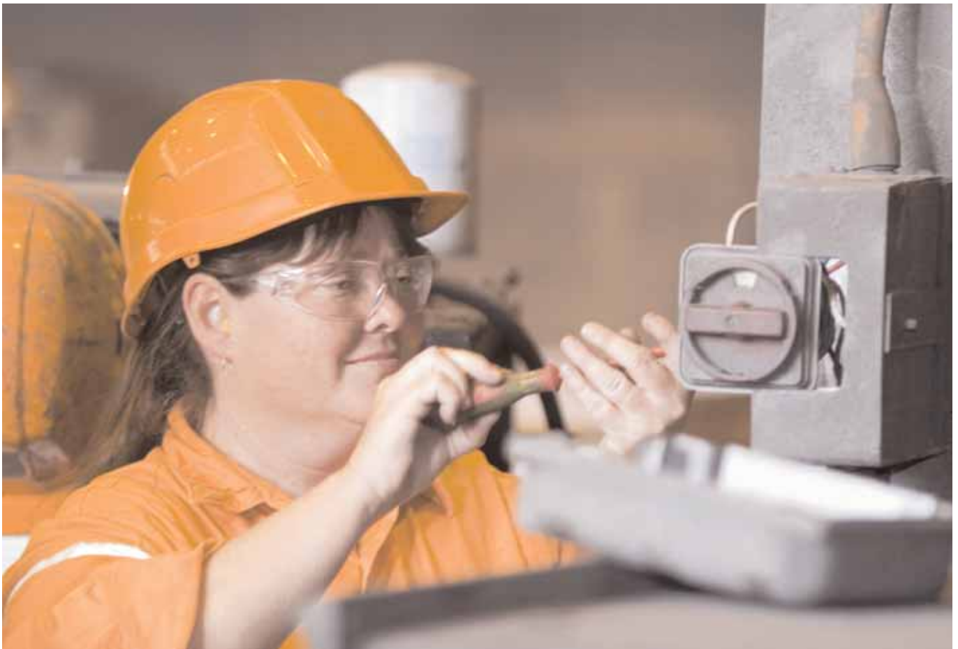
Apprentice Electrician Krystine Cameron replaces a faulty isolator at the Mount Isa copper concentrator
