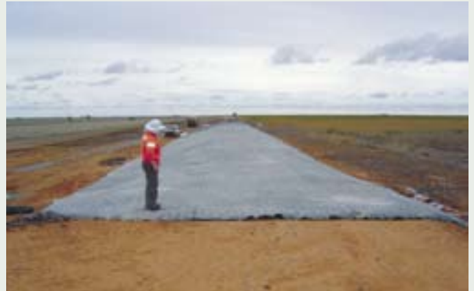
Appropriate construction methods are applied to ensure all tailings management compliance and regulatory matters are met. In 2005 the new northern cell of the tailings dam including spillway upgrade was completed.
