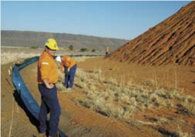
Members of the environment team lead by Mick Hawkins install sediment fencing to minimise sediment spreading from clay stockpile.
