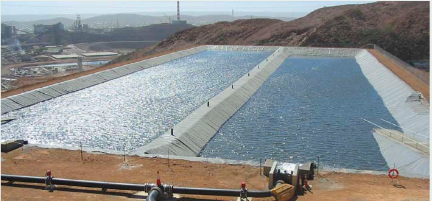
The Rowles Reserve Process Water Dam, built during 2006, is used to store water reclaimed from tailings dams that is then re-used in the copper concentration process.
