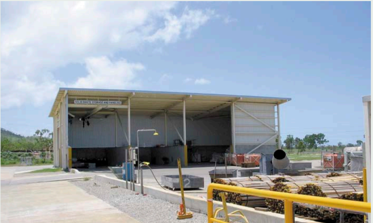
The solid waste storage shed at CRL ensures full containment of wastes through protecting and excluding stored material from the rain and wind.
