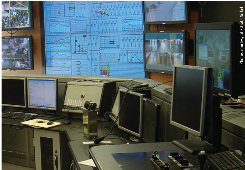
The control room at Xstrata Nickel's Nickel Rim operation
