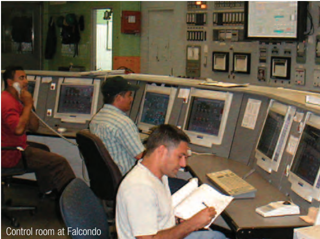
Control room at Falcondo
