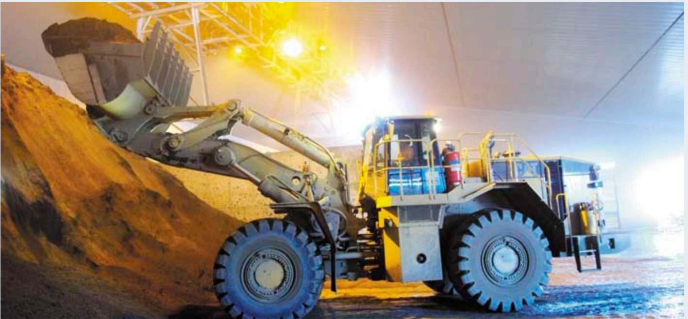
A front-end loader prepares to load zinc concentrate into rail wagons inside the new zinc concentrate storage shed and loadout facility at Mount Isa. The facility was built during 2006 to reduce the amount of zinc concentrate that escapes into the environment during loading.
