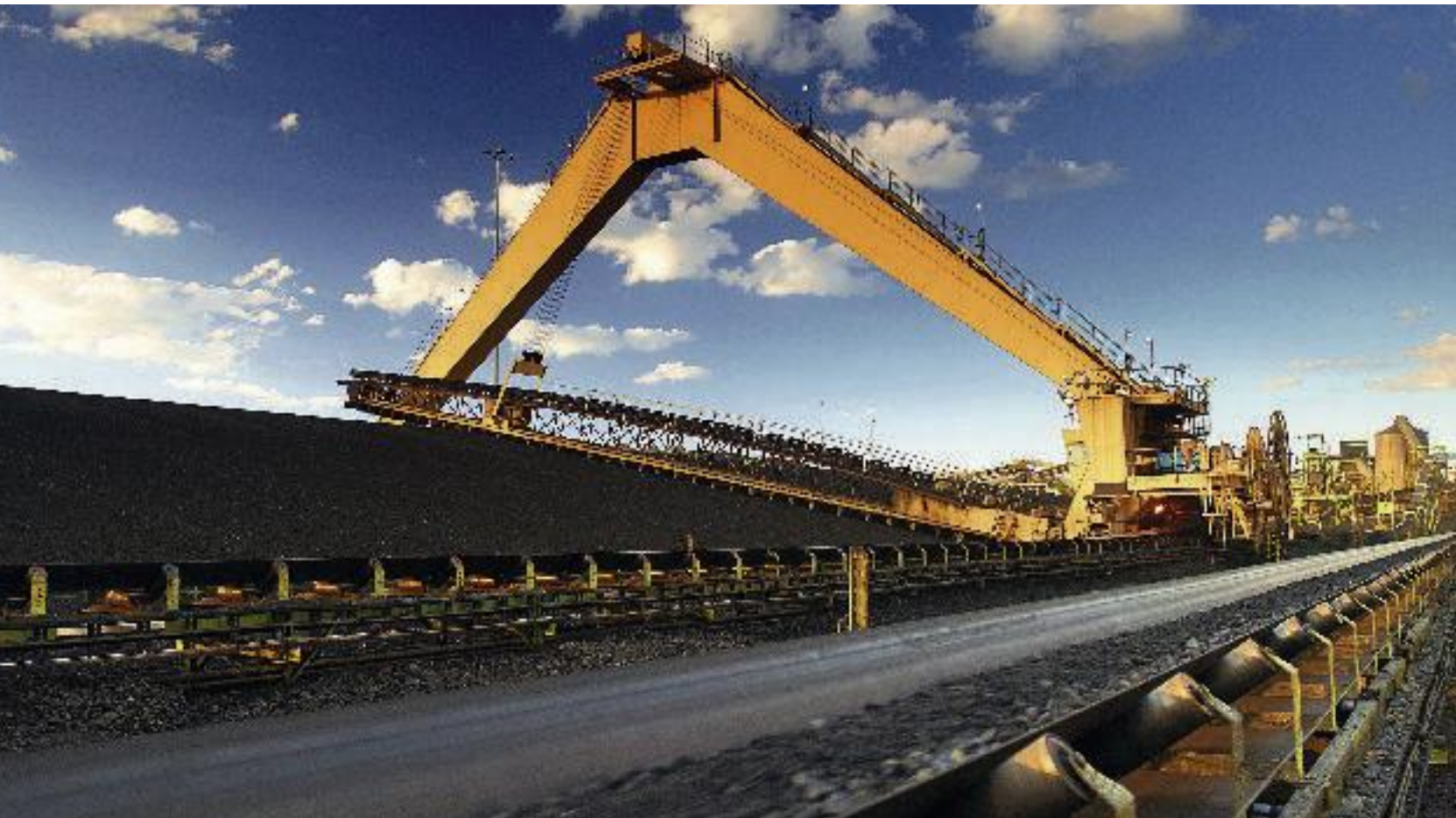
Conveyor belt at Xstrata Coal's Collinsville operation in Queensland, Australia.
