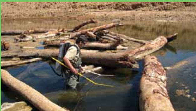
In 2010, MRM installed large woody debris in an additional 35 locations along the McArthur River channel to promote the ecological development of the river system.
